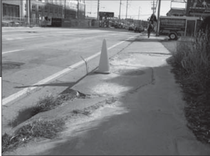
Neglected sidewalks and faded roadway striping
